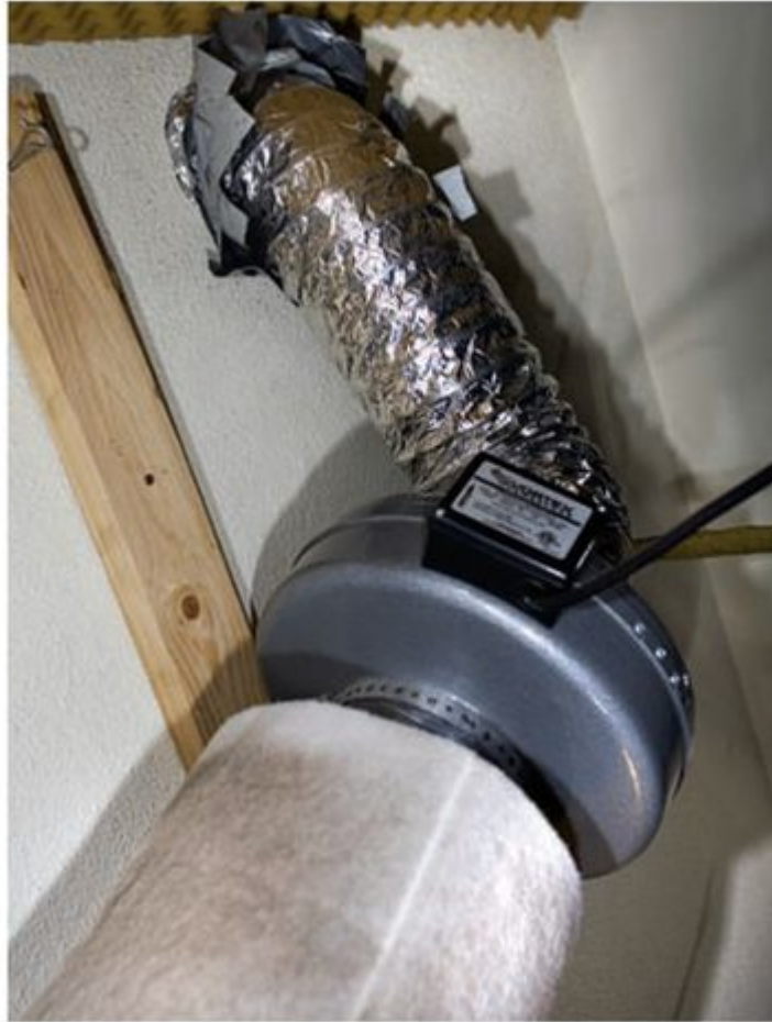
Carbon filters are attached to extraction fans.
